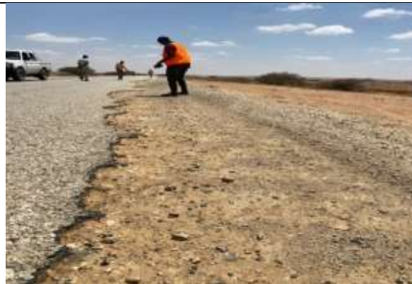
Shoulder erosion picture (RM4) @ Sinujiif-Dangorayo section
