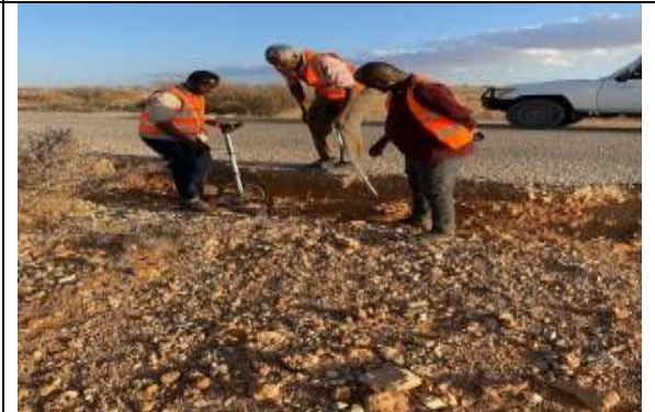
Washed Embankment (RM5) @ Sinujiif-Dangoroyo section
