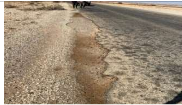
SHOULDER EROSION (RM4) @ GARDO-WACIYE SECTION
