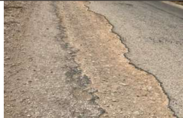
SHOULDER EROSION (RM4) @ GARDO-WACIYE SECTION
