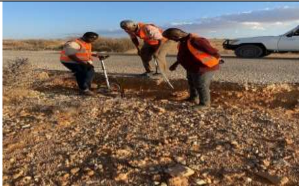
Washed Embankment (RM5) @ Sinujiif-Dangoroyo section
