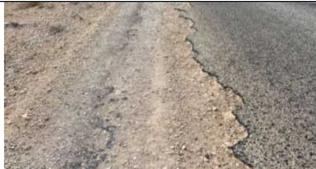
SHOULDER EROSION (RM4) @ ARMO-BOSASO SECTION
