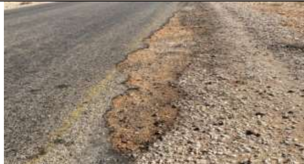
SHOULDER EROSION (RM4) @ ARMO-BOSASO SECTION
