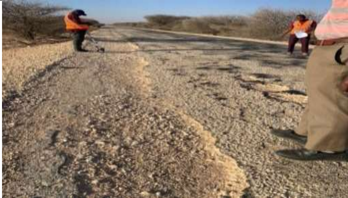
SHOULDER EROSION (RM4) @ HAJI KHAYR-QARDHO SECTION
