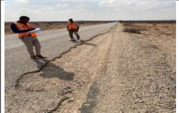
SHOULDER EROSION (RM4) @ HAJI KHAYR-QARDHO SECTION
