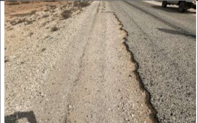
SHOULDER EROSION (RM4) @WACIYE-ARMO SECTION
