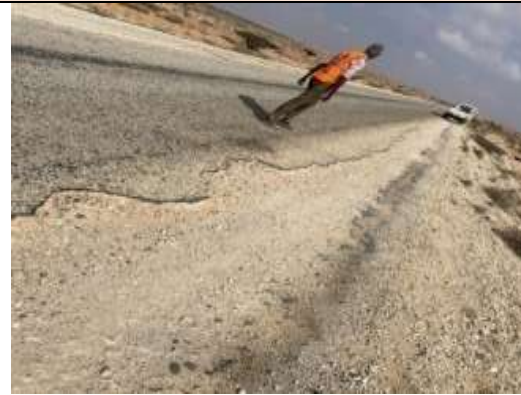
SHOULDER EROSION (RM4) @ GARDO-WACIYE SECTION
