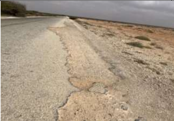
SHOULDER EROSION (RM4) @WACIYE-ARMO SECTION
