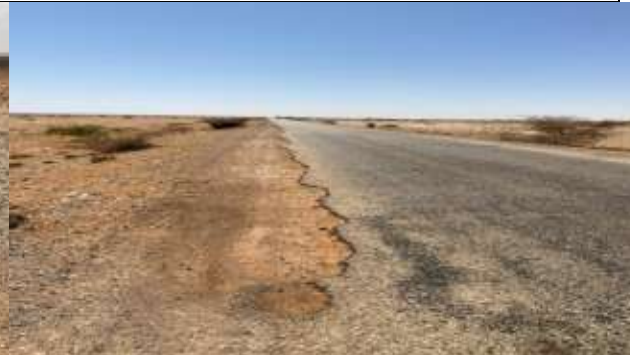
SHOULDER EROSION (RM4) @ DANGORAYO-HAJI KHAYR SECTION
