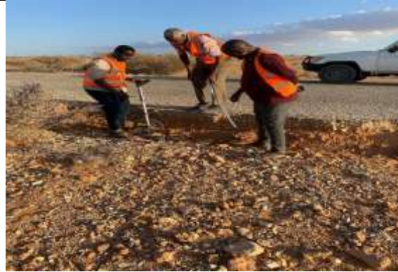
Washed Embankment (RM5) @ Sinujiif-Dangoroyo section
