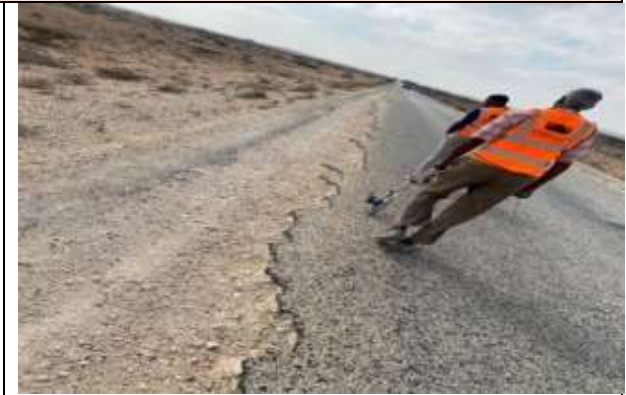
SHOULDER EROSION (RM4) @ GARDO-WACIYE SECTION
