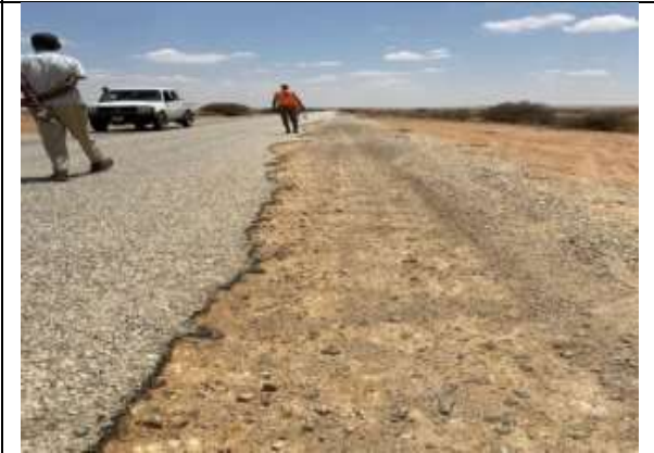
SHOULDER EROSION (RM4) @ HAJI KHAYR-QARDHO SECTION
