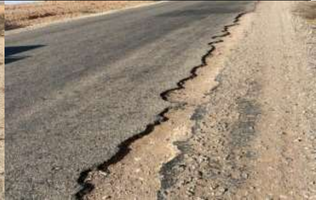
SHOULDER EROSION (RM4) @ DANGORAYO-HAJI KHAYR SECTION
