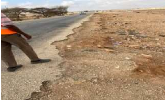
SHOULDER EROSION (RM4) @WACIYE-ARMO SECTION
