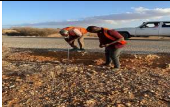
Washed Embankment (RM5) @ Sinujiif-Dangoroyo section
