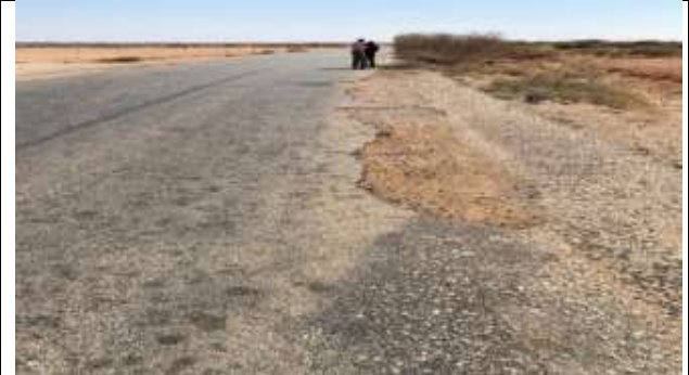
SHOULDER EROSION (RM4) @WACIYE-ARMO SECTION
