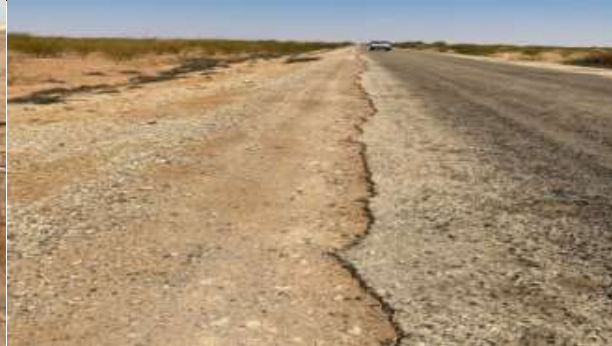
SHOULDER EROSION (RM4) @WACIYE-ARMO SECTION
