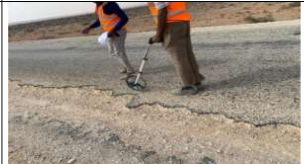
SHOULDER EROSION (RM4) @ ARMO-BOSASO SECTION
