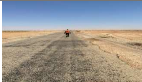
SHOULDER EROSION (RM4)@ ARMO-BOSASO SECTION
