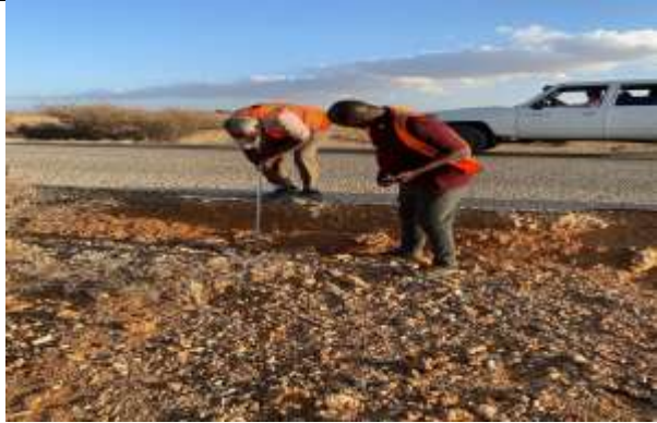
Washed Embankment (RM5) @ Sinujiif-Dangoroyo section
