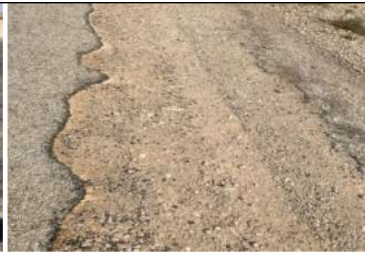
SHOULDER EROSION (RM4) @ GARDO-WACIYE SECTION
