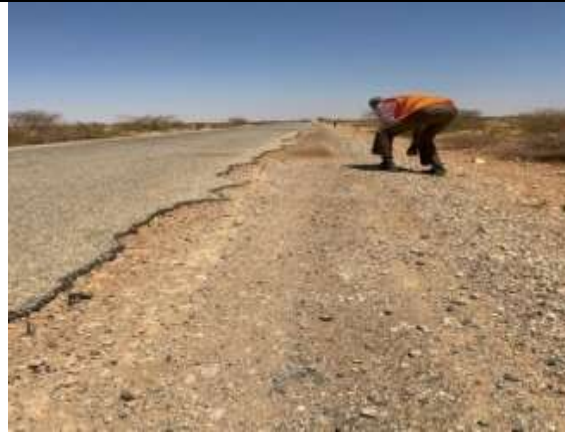
Shoulder erosion picture (RM4) @ Sinujiif-Dangorayo section
