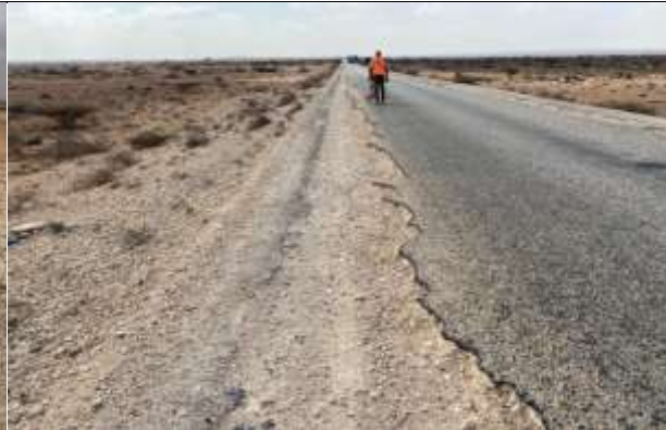
SHOULDER EROSION (RM4) @WACIYE-ARMO SECTION
