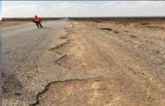
SHOULDER EROSION (RM4) @ DANGORAYO-HAJI KHAYR SECTION
