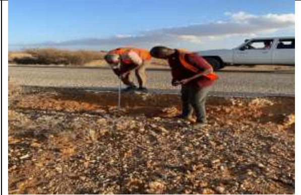
Washed Embankment (RM5) @ Sinujiif-Dangoroyo section
