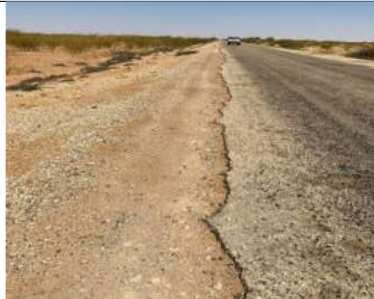
SHOULDER EROSION (RM4) @ HAJI KHAYR-QARDHO SECTION
