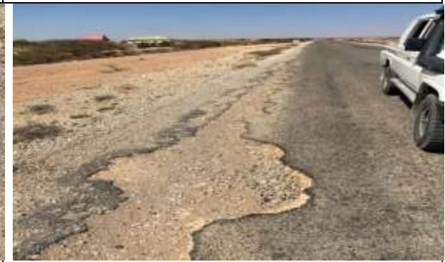
SHOULDER EROSION (RM4) @ GARDO-WACIYE SECTION
