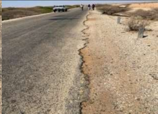
SHOULDER EROSION (RM4) @ DANGORAYO-HAJI KHAYR SECTION
