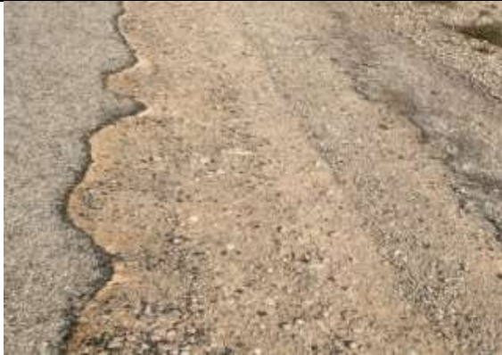
SHOULDER EROSION (RM4) @ DANGORAYO-HAJI KHAYR SECTION
