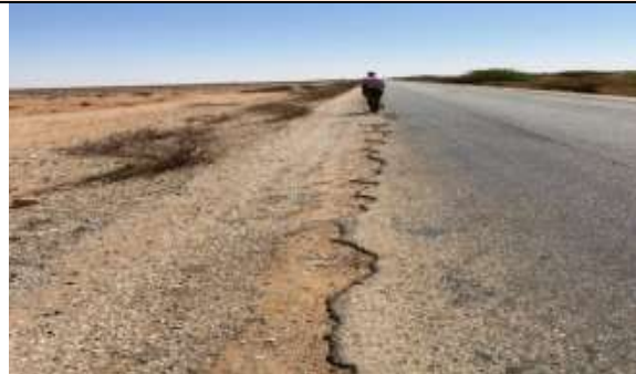
SHOULDER EROSION (RM4)@ ARMO-BOSASO SECTION
