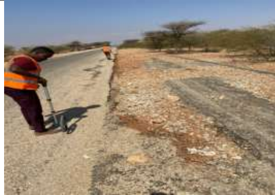
SHOULDER EROSION (RM4) @ HAJI KHAYR-QARDHO SECTION
