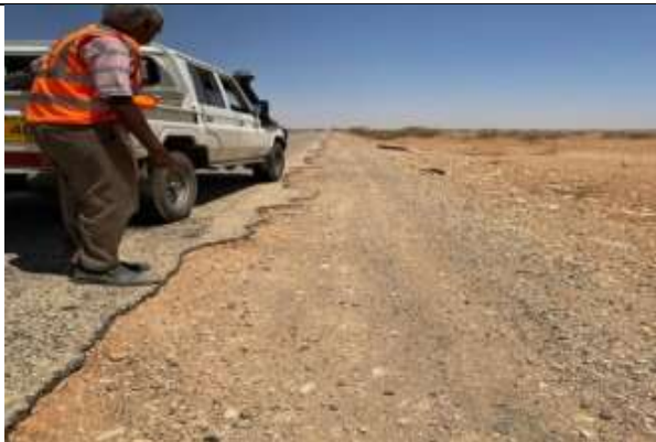
Shoulder erosion picture (RM4) @ inujiif-Dangorayo section
