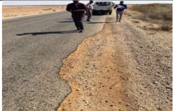
SHOULDER EROSION (RM4) @ HAJI KHAYR-QARDHO SECTION
