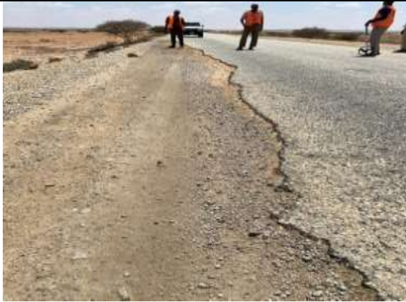
Shoulder erosion picture (RM4) @ Sinujiif-Dangorayo section
