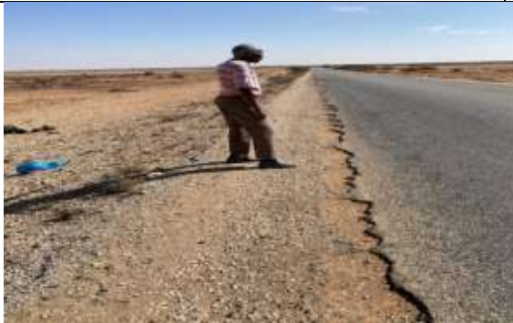
SHOULDER EROSION (RM4) @ DANGORAYO-HAJI KHAYR SECTION
