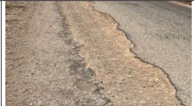
SHOULDER EROSION (RM4) @ ARMO-BOSASO SECTION
