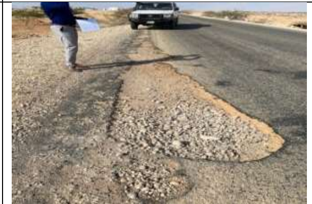
Shoulder erosion picture (RM4) @ Sinujiif-Dangorayo section
