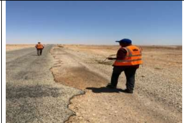
Shoulder erosion picture (RM4) @ Sinujiif-Dangorayo section
